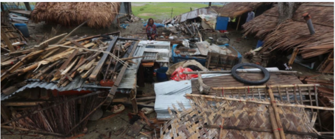
Collapsed houses as Cyclonic storm Fani struck Bidyar Bahon village of Mongla on May, 2019 (Image: Syed Zakir Hossain)
